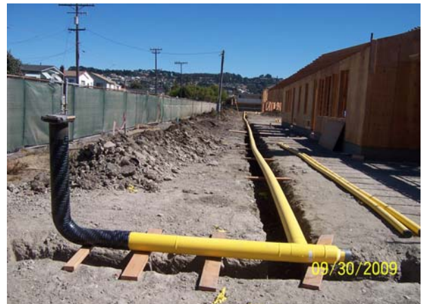
Gas Line at Building Perimeter
